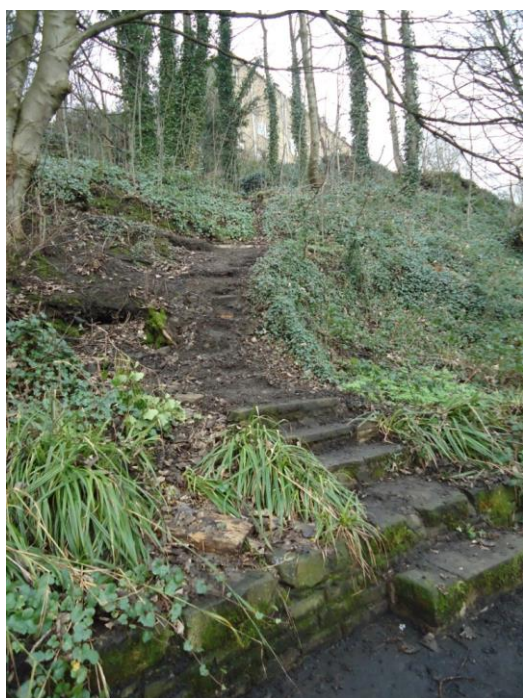
Decayed steps in 2016
